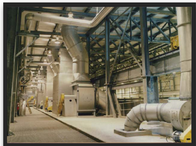
HOOD EXHAUST SYSTEM
